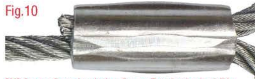
PVC Swage Cover is missing. Swage Termination is visible.
